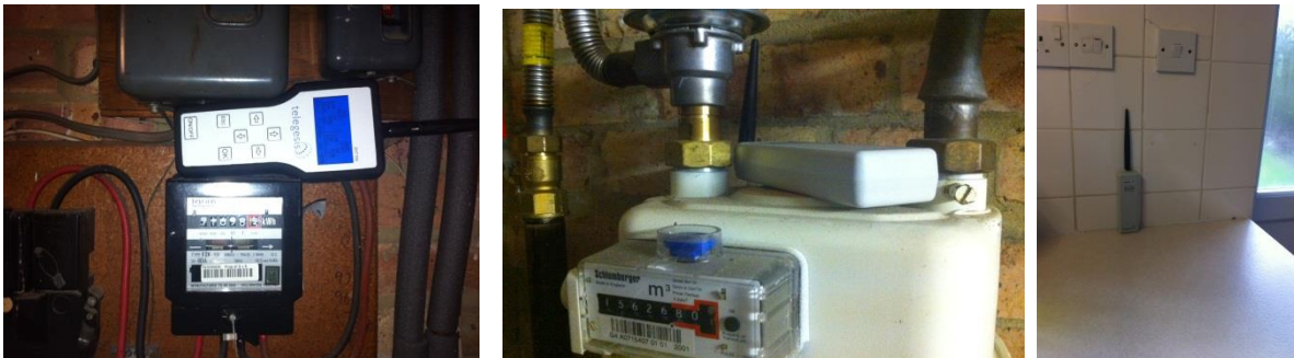
Figure 35: RangeFinder locations: Electric meter, Gas meter and Kitchen work surface
