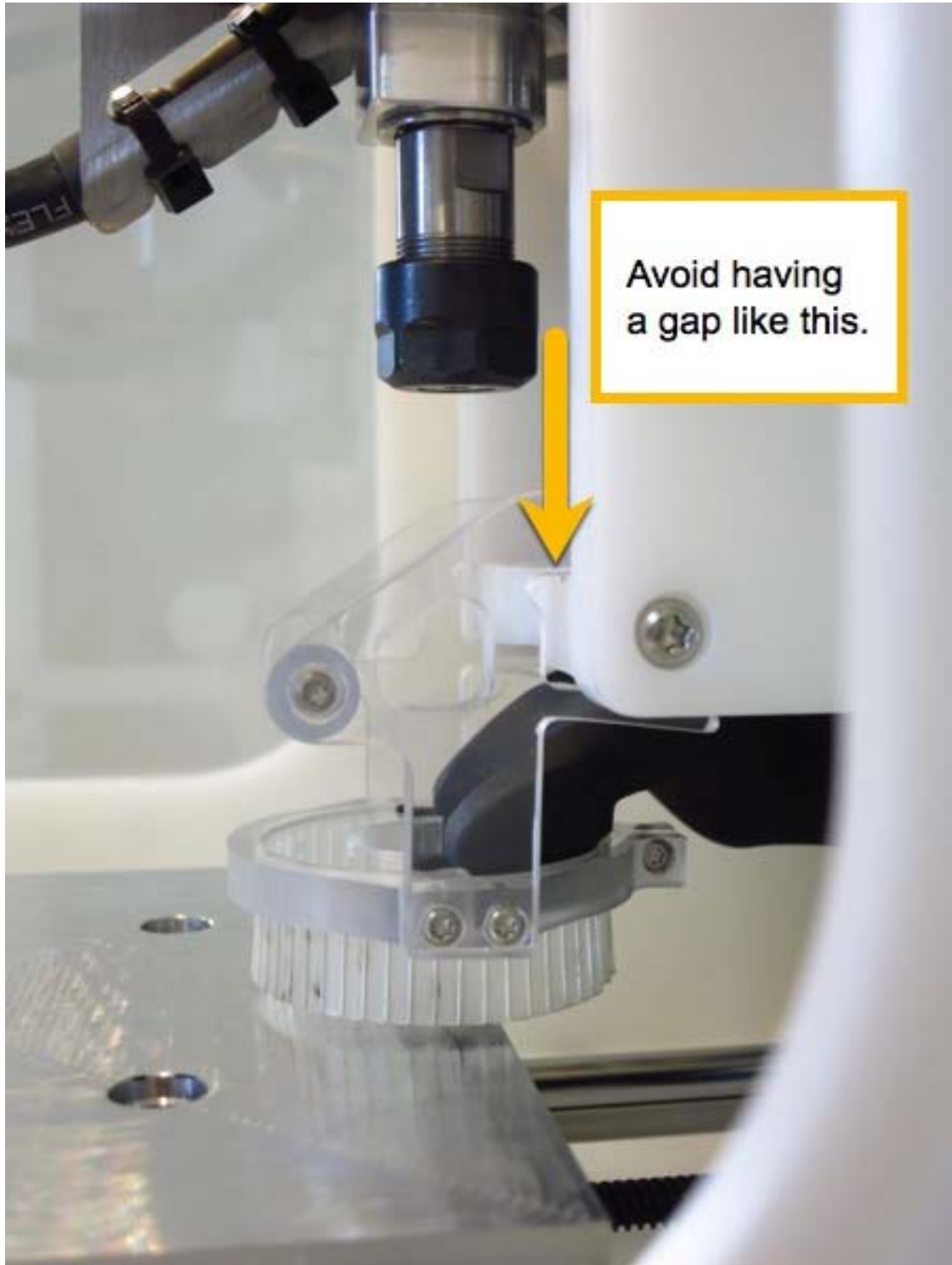
Incorrectly installed Dust Collector Hood: Avoid having a gap between Dust Collection Hood arms and X Carriage frame
